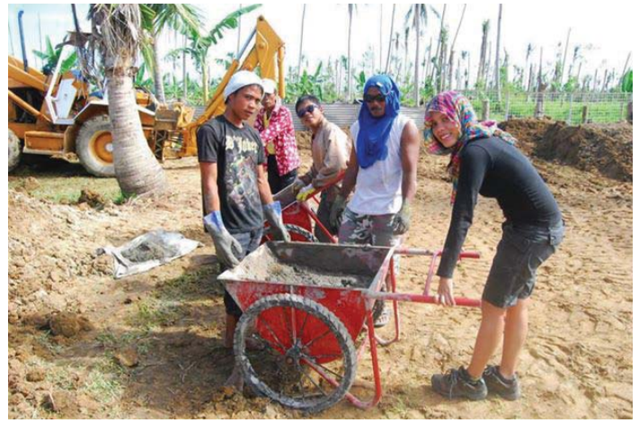
Gloryrose Dy joins Earth Village Project in creating an Earthship Biotechure in Barangay Batug, Dulag, Leyte, one of the areas which survived Typhoon Haiyan. Switotwins, Inc. is currently drafting an architectural tour on alternative construction to be set in Dulag, Leyte.
