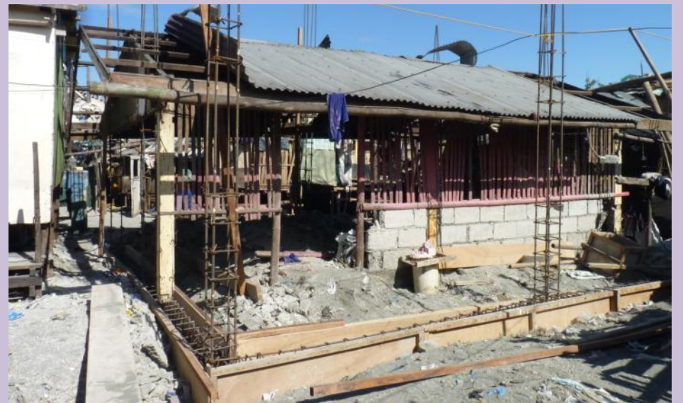
Foundations have been set for the new multi-purpose center with the existing community center being dismantled at the background.
