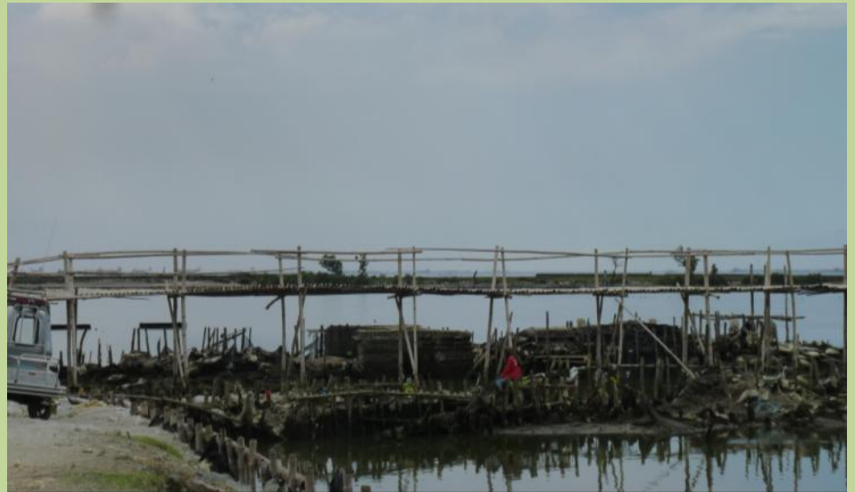
Constructed over the earth dike and over 300 meters long so far, the bamboo bridge was elevated up to 3 meters high for Pulo residents to safely cross during high tides.
