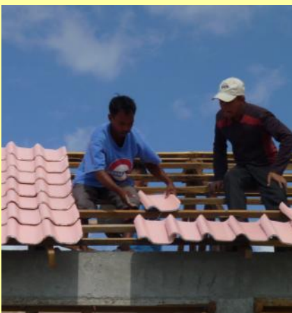
Top: The elevated livelihood center will store supplies of rice and fishing nets; Workers construct the framing for the installation of micro-concrete roofing (MCR) Bottom: Architect Cesar Aris of FDUP supervises the laying of MCR tiles.
