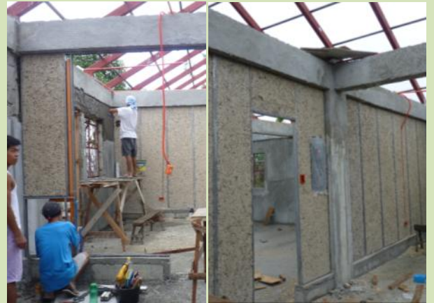
Top: The multipurpose center was built just behind the Suburban covered court that serves also as temporary evacuation center for the community. Bottom: Wood-wool cement boards are used for the walls.
